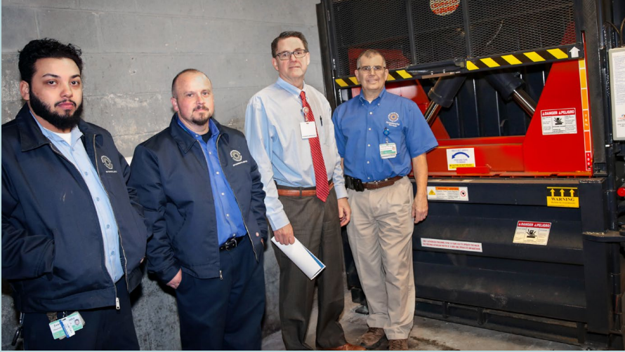
Baler for the new blue wrap recycling program at Rhode Island Hospital
